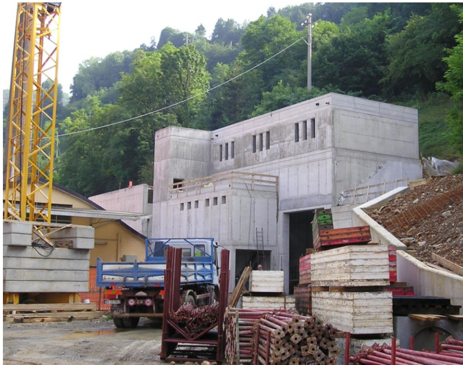
Fig. 6. – Casnigo power station.
