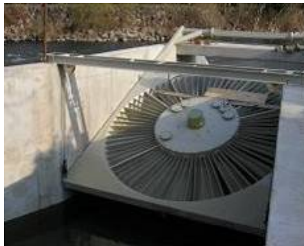
Fig. 6. Example of VLH installation.
