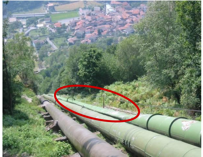
Poor maintenance procedures for the air vent
