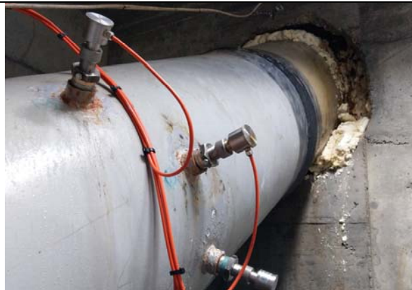
Selva Gardena HPP – differential detection system (D=1)
